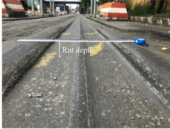
Figure 1.1. Rutting distress on entrance street of Cat Lai port, HCM City (taken in July 2021)
